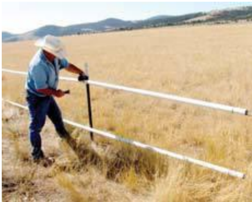
Figure 11: Installation of crossing structure: Note the plastic pipe slipped around the top and bottom wires Montana FWP
